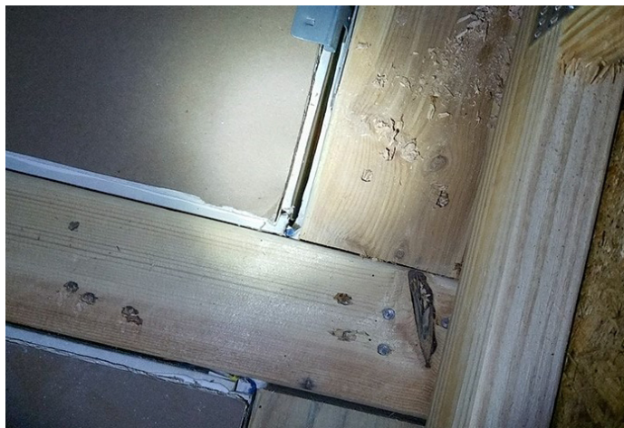
View from attic showing gap between drywall and top plates at interior and exterior walls
