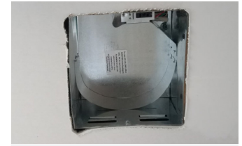
Gaps around bath exhaust fans
