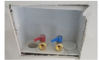
Gaps around washer/dryer, refrigerator and stove casings
