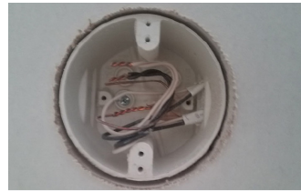
Gaps around all ceiling penetrations
