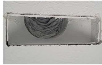
Gaps between HVAC boots and drywall
