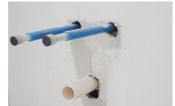
Plumbing under vanities and at water heater must be sealed at drywall
