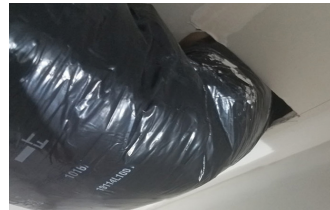
Mechanical room penetrations must be sealed with caulk or foam, NOT insulation
