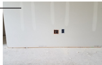
Drywall held loosely to bottom plates with only 2 screws across 5ft section
